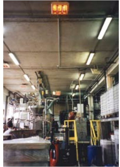
IRCF is often installed in large warehouses. They give instant and effective heat which makes them profitable quickly.
