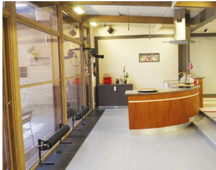
Installed by a window the ribbed pipe radiators effectively counteract cold draughts that frequently form by large glazed areas.
